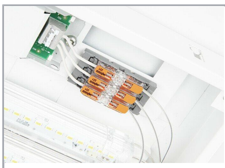
Multi-pole, fixed lighting fixture wiring
